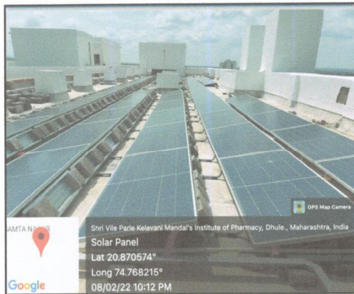
Photograph of Roof Top Solar PV Plant:
